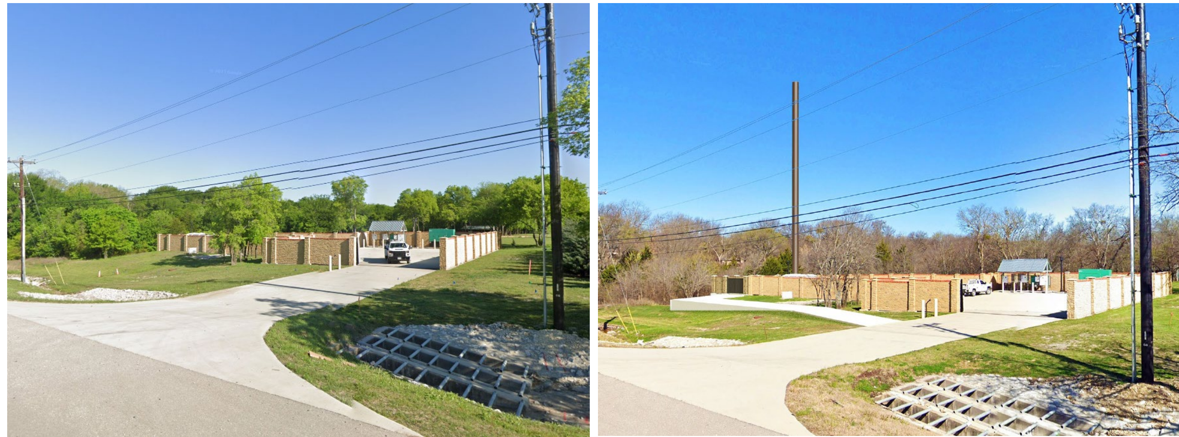
Attachment: Staff Presentation (Anthemnet - Frontier Lift Station Cell Tower - Specific
