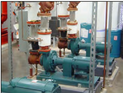
Mechanical Noise Control
